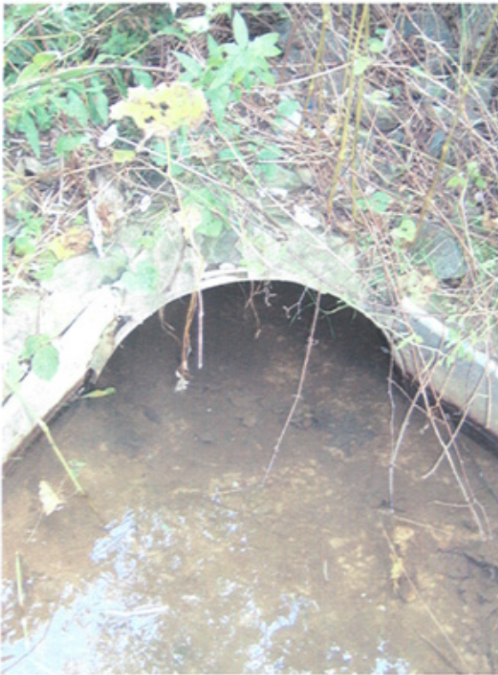
24" CMP with bottom 8' sediment covered
